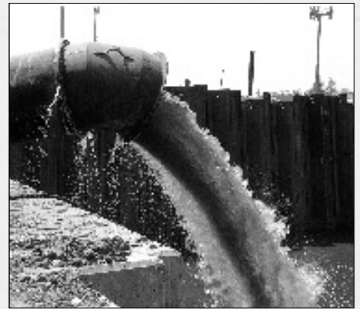
Pump test at the 17th Street Canal. Photo: Moving Water Industries
